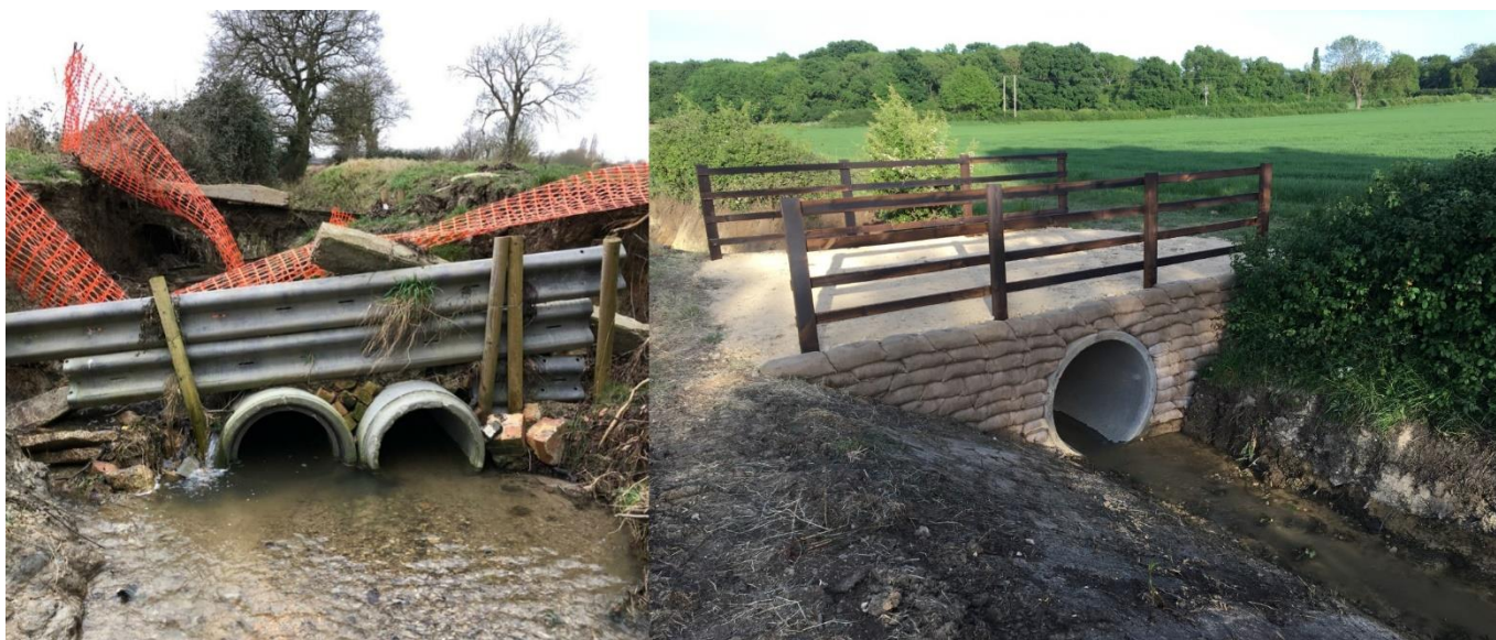
Figure 7-3 Culvert collapse and subsequent on Marholm Brook
